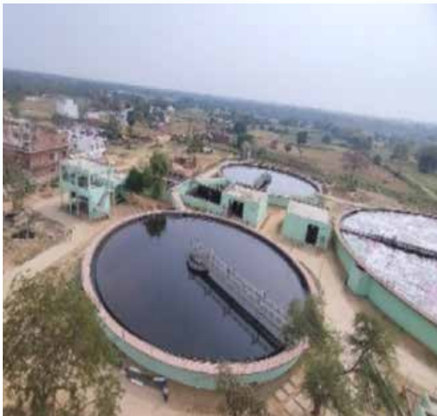
Interception & Diversion works and 30 MLD STP at Jaunpur completed. The project taps sewage through 14 nos. of I&D structures to abate the pollution of the river.
