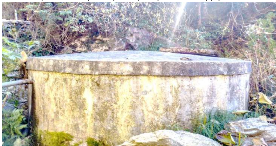
Figure 4.19: Closed tank to supply drinking water, Uttarkashi SC division
